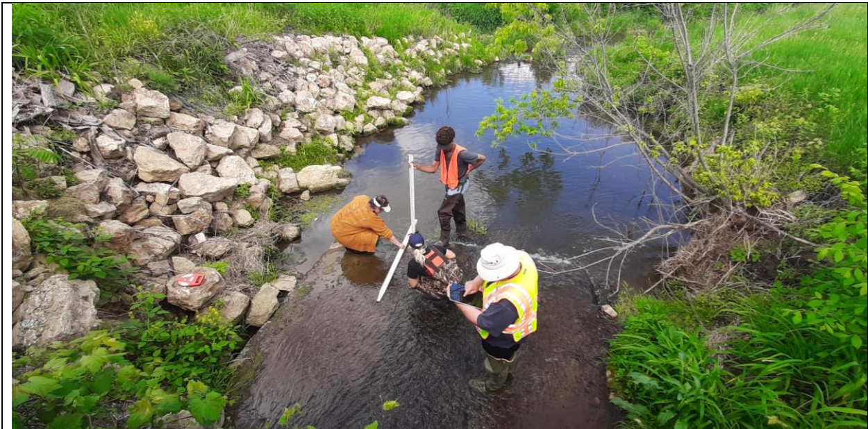
Beginning in 2021 and continuing in 2023, the Monroe County Land Conservation Department is conducting a Road Stream Crossing Inventory and Assessment with the assistance of the Wisconsin Department of Natural Resources and funding from Trout Unlimited and the Federal Emergency Management Agency. The Inventory & Assessment project has evaluated nearly 550 road-stream crossings throughout Monroe County, including the Little La Crosse Watershed, for fish passage and flood resiliency using criteria from the Great Lakes Stream Crossing Inventory.
