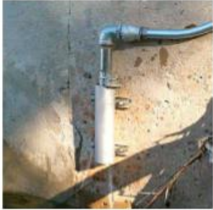
Flood sensor mounted on bridge.
