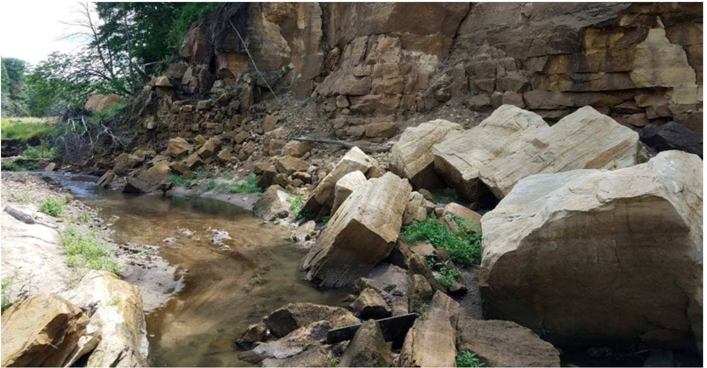
One of the breached dam sites in the Coon Creek Watershed. Photo by Eric Booth
