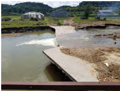
Farm structures such as this stream crossing are some of the most frequently damaged assets during storm events.
