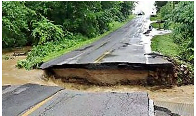
Future infrastructure can include updated standards reflecting the likely size of future events, and incorporating both “gray” and “green” design features.
