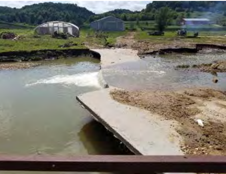
Farm structures such as this stream crossing are some of the most frequently damaged assets during storm events.
